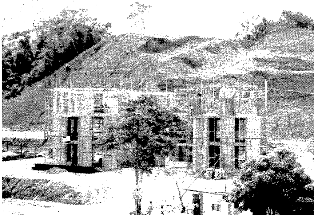
The new library for Antillian College is now under construction in a valley that workers filled with a mountain.
