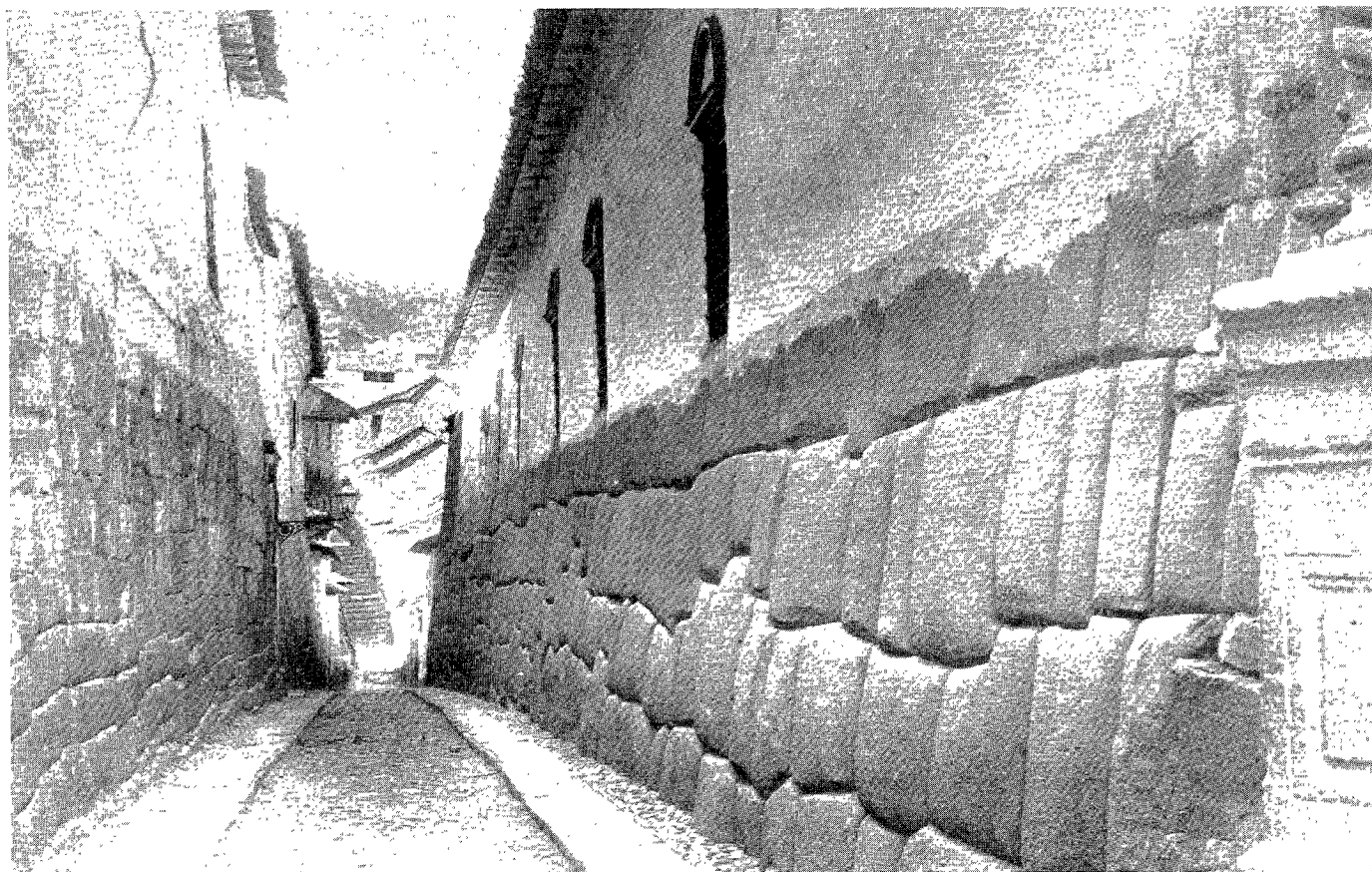
In an area where earthquakes frequently destroy modern masonry, Inca stonework, such as this building foundation in Cuzco, has stood for centuries. "Come, and let yourselves be built, as living stones, into a spiritual temple," Peter wrote in 1 Peter 2:5, N.E.B. The divine Mason is able to take multisided Christians with their unique talents and personalities and shape them into an indestructible, living temple.
