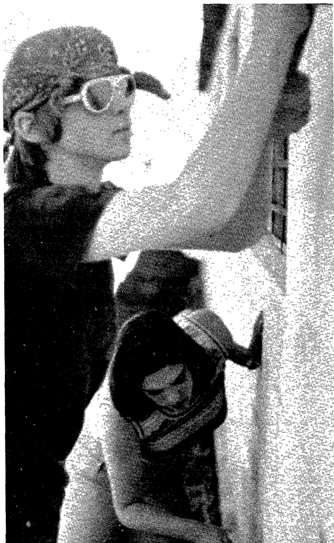
Students from PUC Preparatory School traveled to Tezopaco, Mexico, to improve the appearance of a clinic. They painted the walls white.
