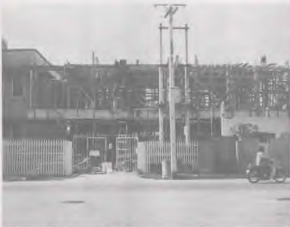
Construction of stage 1 of Haadyai Mission Hospital expansion programme to be completed in June, 1981.
