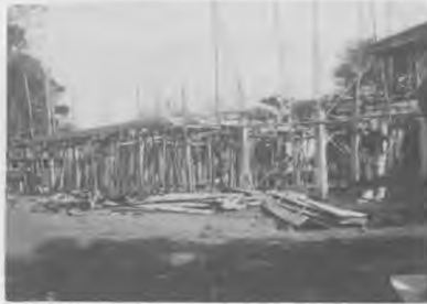
Pastor Art Bell, Administrator of the Thailand Educational Center, stands at far right in front of the new boys' dormitory that is under construction.
