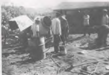
The cement mixer always seemed to be a focal point of activity. In the background is the Educational Centre Church.
