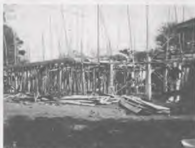
Pastor Art Bell, Administrator of the Thailand Educational Center, stands at far right in front of the new boys' dormitory that is under construction.
