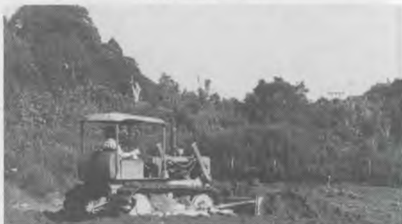
Bulldozer rebuilding the Ayer Manis airstrip and leveling the building site of the new hangar to be constructed there this year, 1986.
