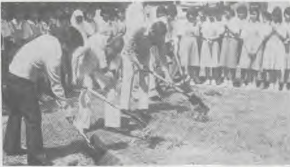
Tan Sri Datuk Amar Sim Kheng Hong with garland, minister of finance led out in the ground breaking.
