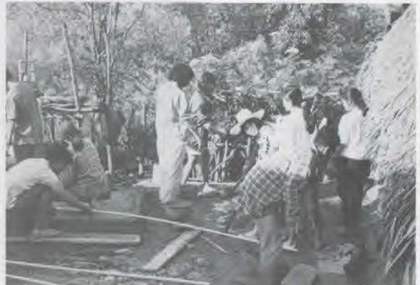
BAH nursing students help to build sanitary facilities in the Hmong village of Doi Sang.
