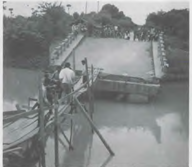
Many roads were damaged or destroyed by recent floods.
