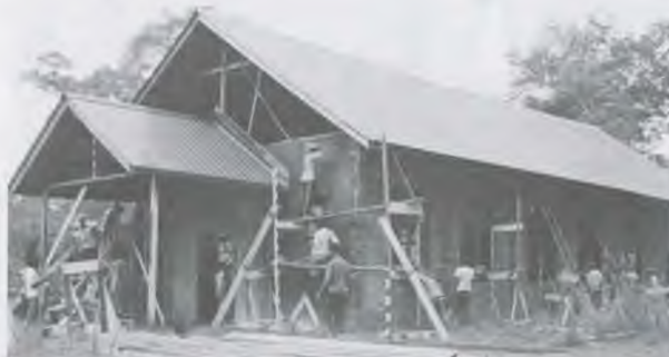
In addition to their offerings, church members in Ampungan donate their Fridays and Sundays to the completion of a new church.
