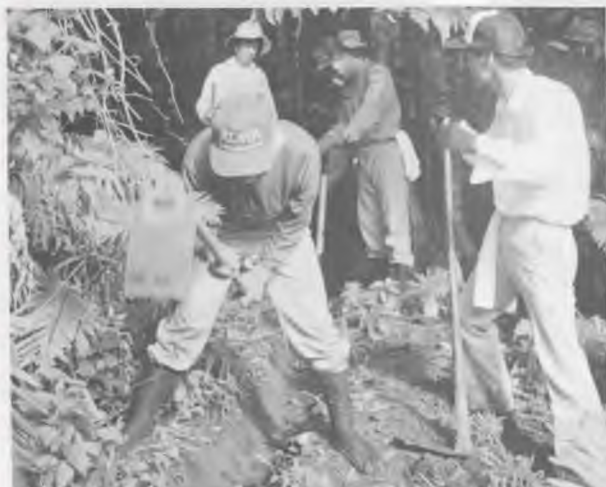
ADRA Japan team digging ditches to lay pipelines at Toviu and Lomou.
