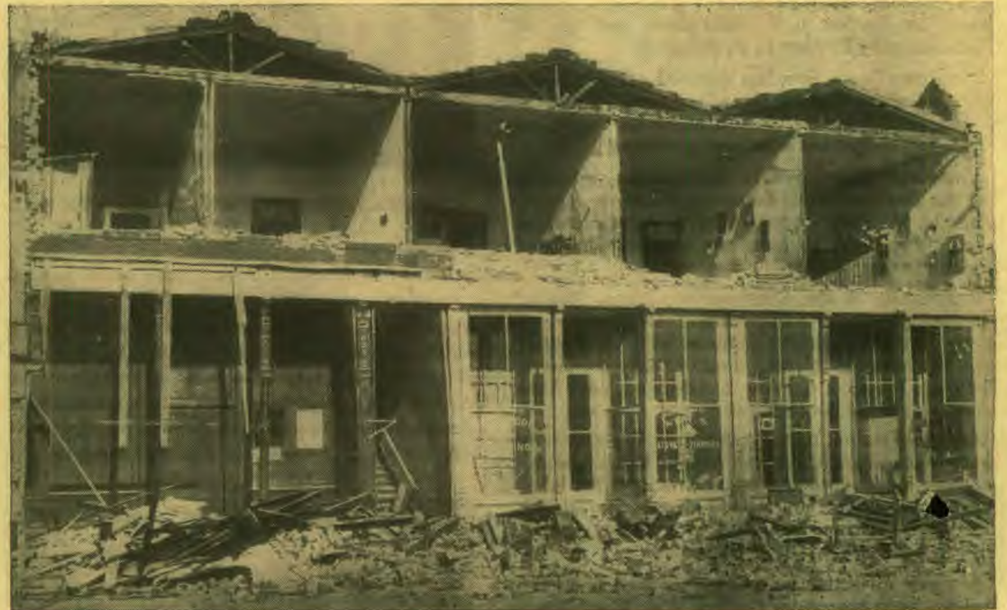
Gobbi Building, Healdsburg. This is a typical scene which might be met in every town where the earthquake did any considerable damage, the front wall fallen away, leaving open bedrooms which appear like little doll houses seen on exhibition.
