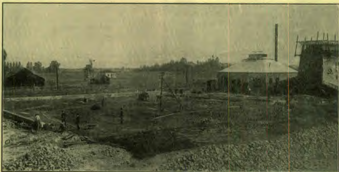
The Pacific Press grounds, Oct. 9, 1906, prepared for cement floor and frame, looking from the boarding house, where the offices now are, northeasterly. The power house and tank house to the right.
