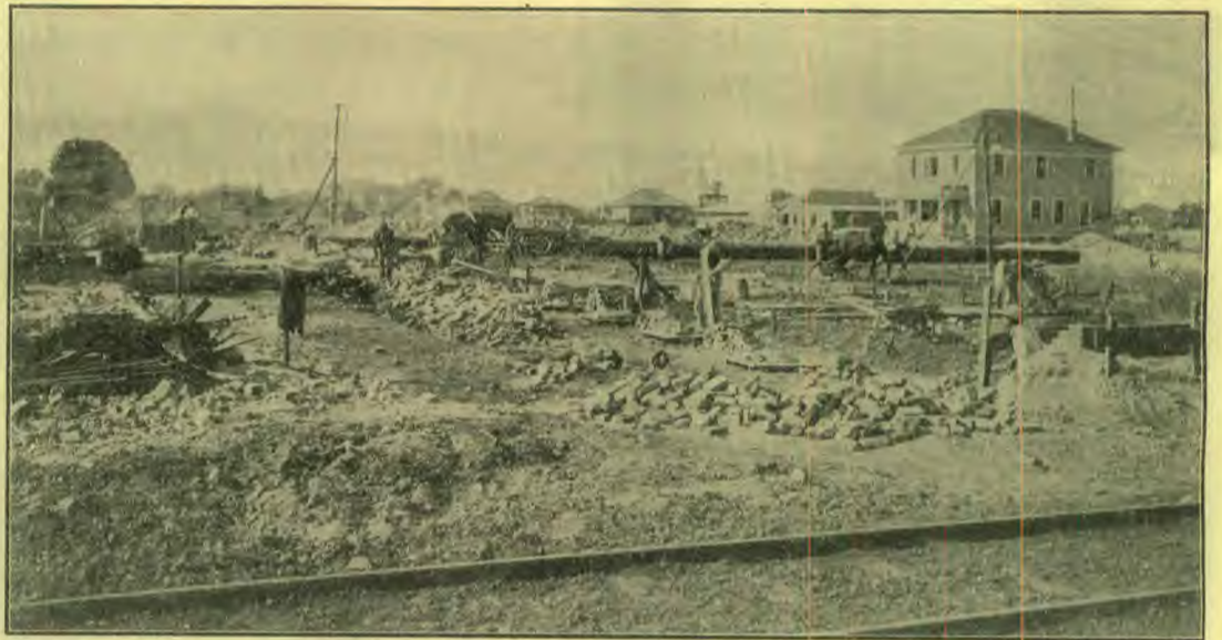
Looking from the northeast on the railway, Oct. 9, 1906, across the building site of the Pacific Press, now cleared of debris. The x in the foreground at the right marks the new foundation wall. The o near the middle foreground is where the old wall stood. A large strip has been cut from the east side. The boarding house and temporary plant in the distance.
