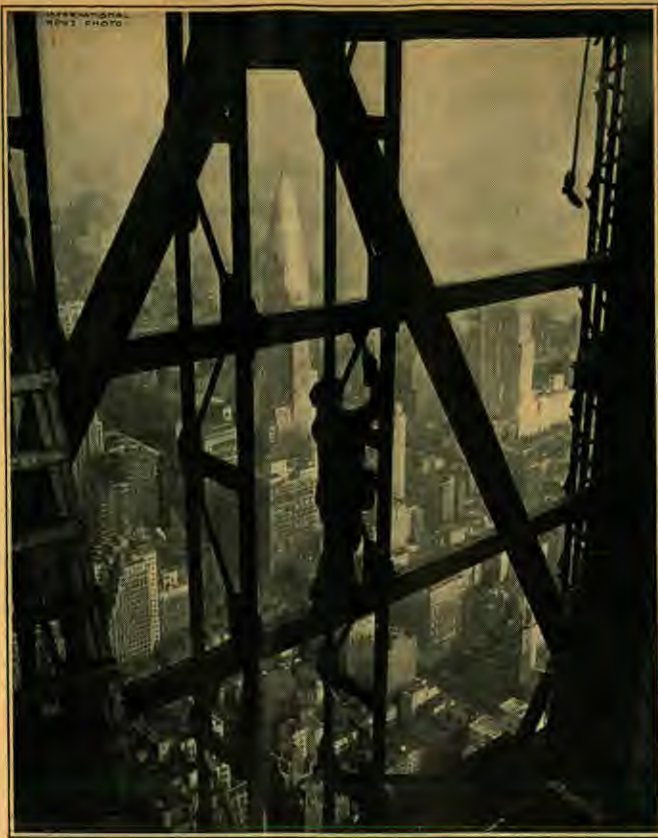
The skeleton of a skyscraper aptly illustrates the vast importance of iron in our modern civilization.
