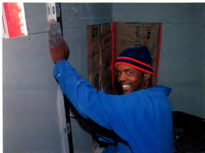
Bertham Rosebert, a contractor, was one of 16 volunteers from the South Park church in Birmingham, Alabama. He is measuring sheet rock while repairing a Katrina-damaged home.
