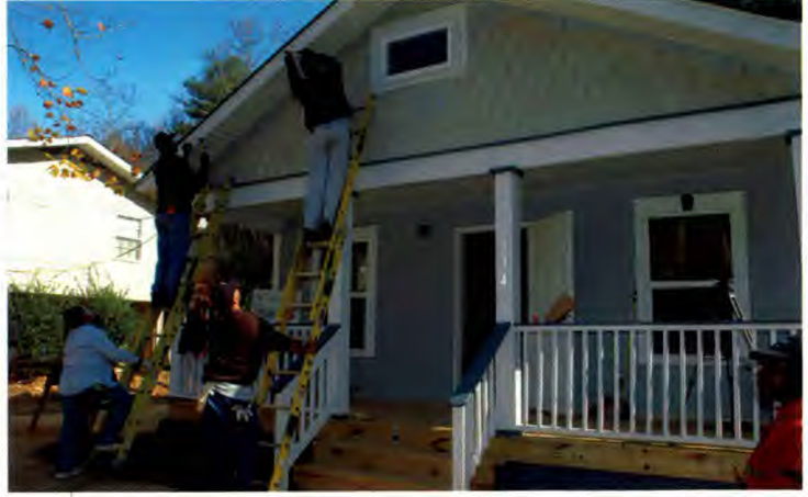
After seven Sundays of work on the Habitat for Humanity house in Atlanta, finishing touches were completed before the dedication ceremony.
