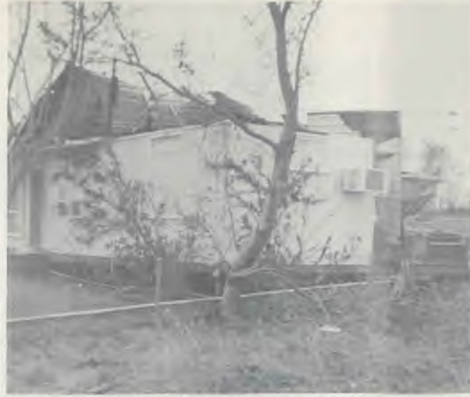
This house is typical of many that were extensively damaged by the force of the cyclone.
