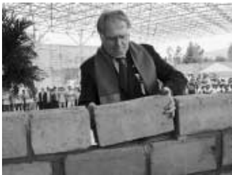
Pastor Paulsen lays a symbolic brick in the construction of a multifunction complex at the Bolivia Adventist University, perhaps the largest Adventist higher-education centre with some 6500 students.
