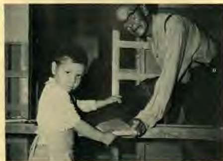
Randy Johnson, three years old and the youngest member on the construction crew is holding a board while Ambrose Herkimer uses the saw skillfully. Brother Herkimer is eighty years old, and is the head deacon. He amazes everyone as he joins in and helps.
