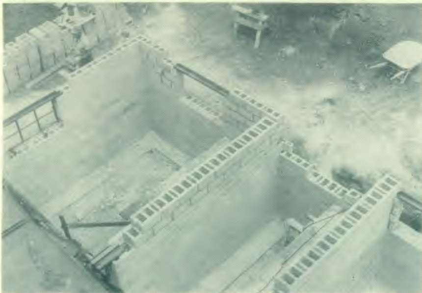
Aerial view of construction on boys' dormitory at Enterprise Academy. The new addition will provide student rooms to replace those destroyed on the third floor and will house new bathroom facilities.
