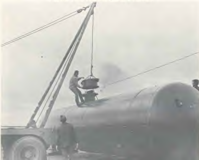
Storage tank for fuel given to mission.
