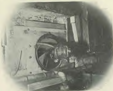
One of the ventilating-fans being installed in the factories and workshops throughout the city.
