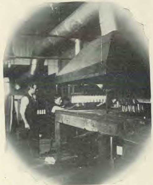
Hood for drawing off gases generated in the process of manufacturing gas mantles, installed upon advice of the health department.
