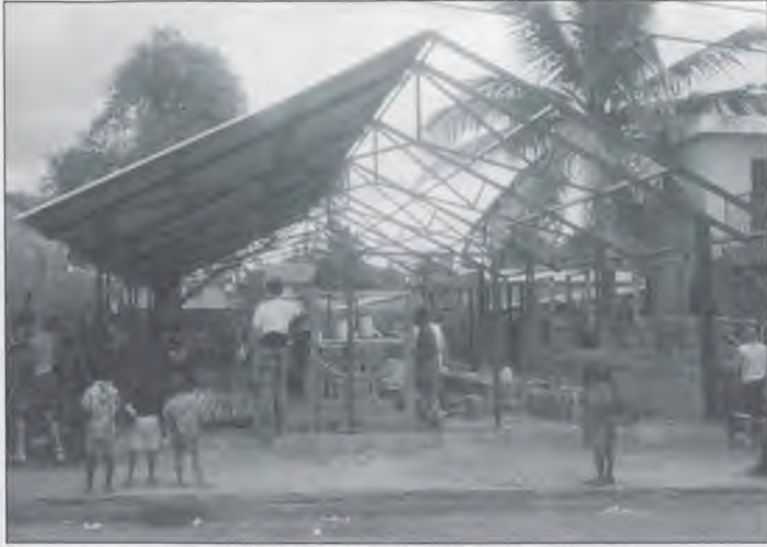
The 19 Indiana Academy seniors and a handful of adults were instrumental in the construction of this new church in Bani, Dominican Republic. "We support missions and service to others," says former Principal Nick E. Minder.
