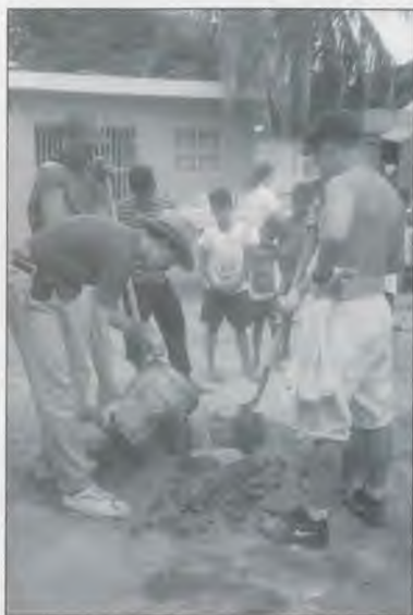
After the cement mixer broke, the Indiana Academy team improvised by digging holes and mixing the cement by hand.
