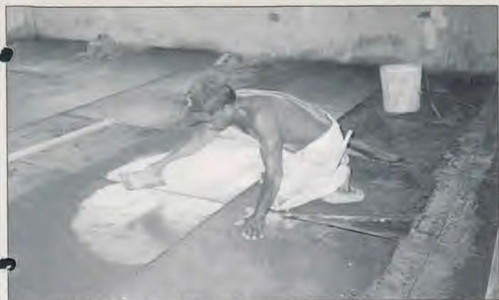
A local workman puts the finish coat on the floor in one of the Maranatha Escuela classrooms.
