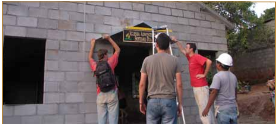
Adam Shull and Eric Shull hold the new Seventh-day Adventist Church sign in place as it is secured.
