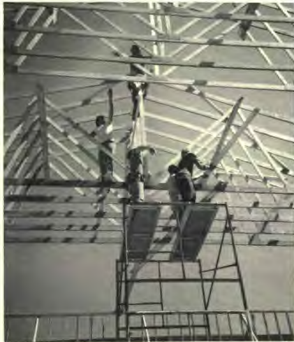
The assembling and placement of the trusses required the cooperation of many workers.
