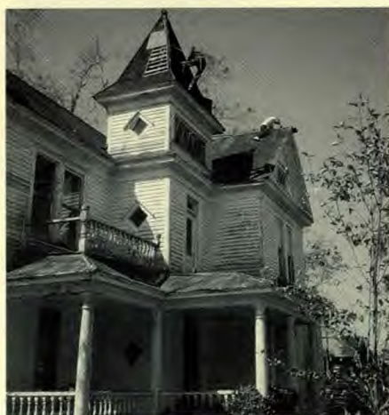
Nels Angelin (on cupola) and Dale Collins (on ridge), Collegedale church members, made temporary repairs to the roofs of many homes in Bishopville. The van was one of two lent to the relief project by Southern College.
