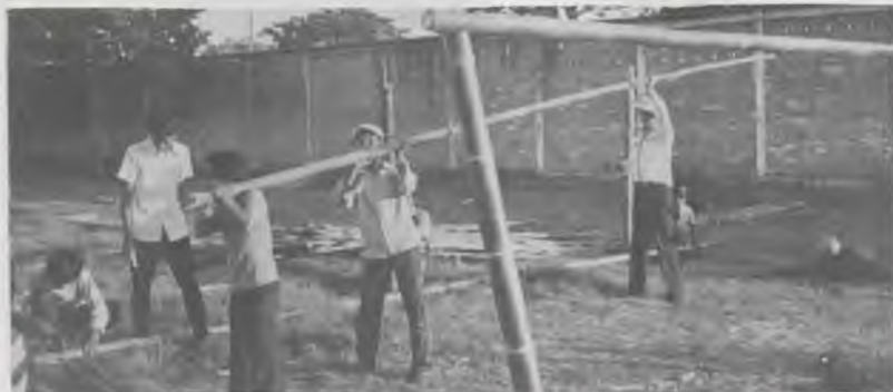
Pastor Bassham and his Ministerial Students begin construction on their booth for the Chiangmai Winter Fair.
