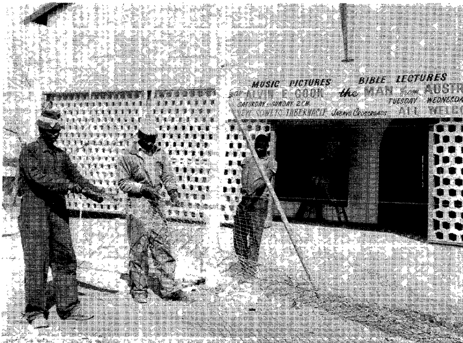
Workmen busy getting the Soweto Evangelistic Centre ready for the opening of the campaign there.
