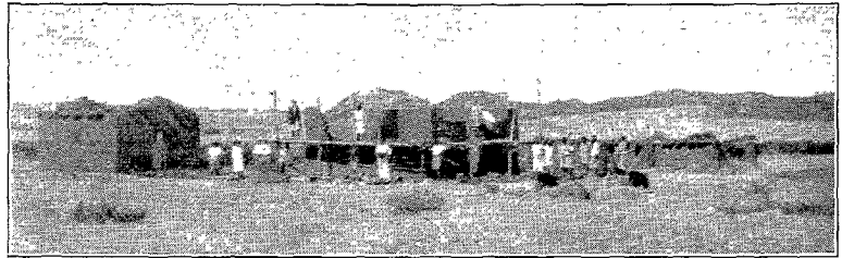
Girls' School, Ntusu, in course of erection. Miss L. Clarke is taking charge.
