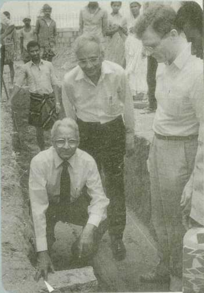
Foundation stone laid by G J Christo for the Division office, Hosur, April 1987, R D Riches and Koilpillai look on.
