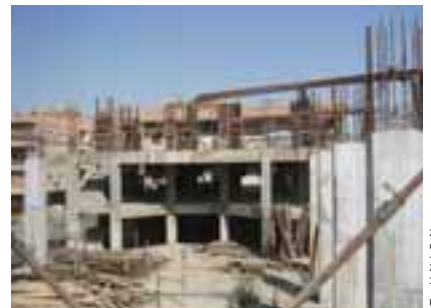
NEW CHURCH HEADQUARTERS: A building being constructed next to the Adventist church in Baghdad will be the new home of the Adventist Church headquarters in Iraq.
