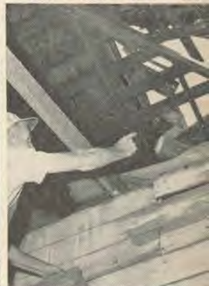
This man points to the hole in the roof wrecked by the explosion. It is dangerous to make moonshine and to drink it.
