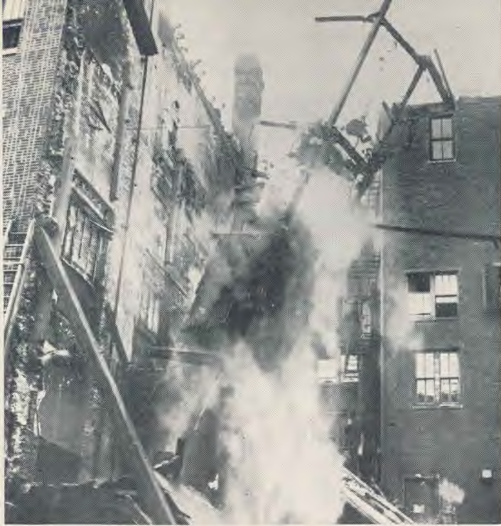
Pickwick's elevator goes on its last trip when standing portions of the building are razed to prevent collapse.
