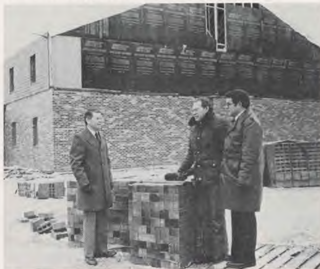
Inspecting the Moberly building progress are (from left) Jim Culpepper, Pastor Harry Reile, and Mike Foxworth, head elder.
