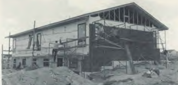
The new church school building in Green River, Wyoming as it nears completion.
