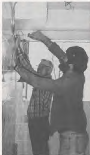
Roger and Doug Eno do electrical work in the shower room of the girls' dorm.
