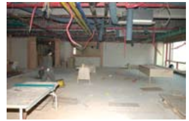
It may look like a bomb has exploded, but this is the beginnings of the new church. Bare floor and walls, but not for long.
