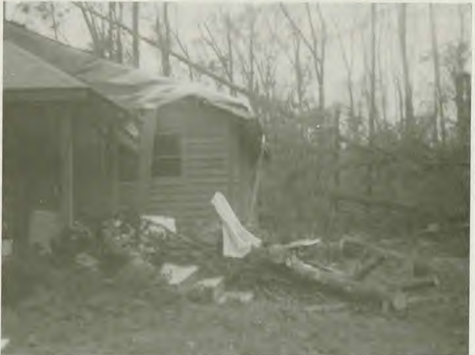
A partial view of the devastating effects of Hurricane Hugo on one home in South Carolina.
