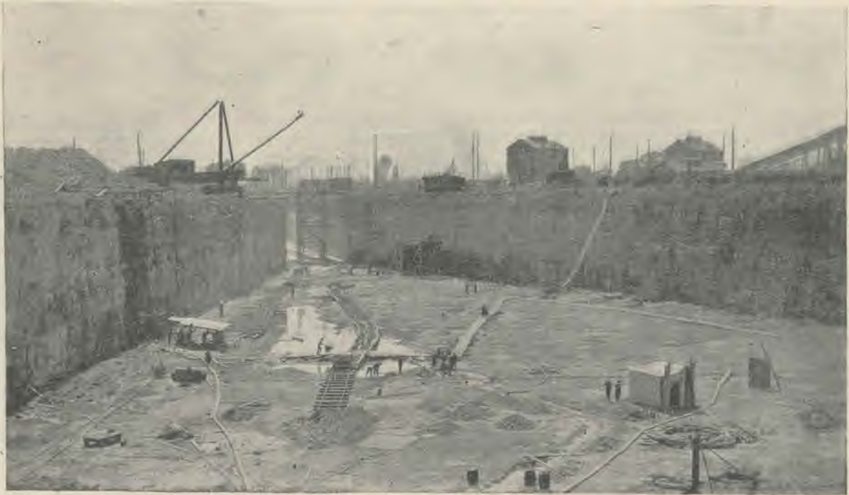
Fore Bay, Chippawa Development of Ontario Hydro-Electric System
