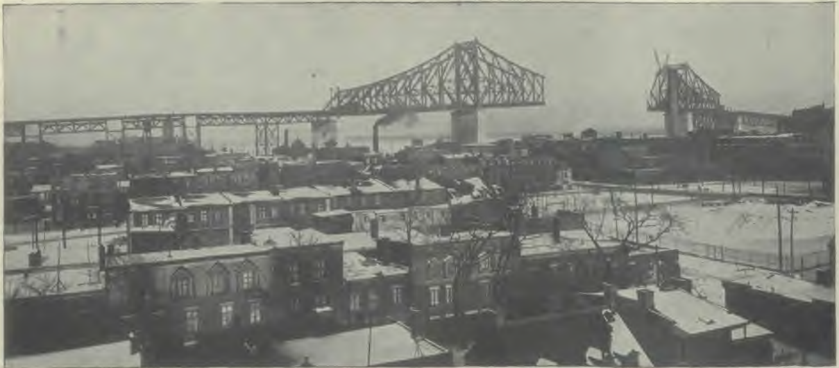
The new Montreal-South Shore bridge which spans the St. Lawrence at Montreal, between Quebec province and the United States, thus speeding up traffic. The bridge will be more than a mile and a half long when the central span is lifted into place.
