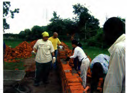
Rhonda Maddox (left), Winston Mills, and Joy Searcie busy at constructing the fence.
