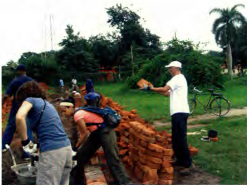
Walter Fordham (left), and Brenda, Kristen, and Keith Wood work on constructing the fence.
