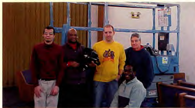
Mike Sommersell Jr. (left); Mike Sommersell Sr.; Jon Weigley, assistant pastor; Vernon Taylor (kneeling); and Steve Hamilton stand in front of the 30' lift used to install new lighting in Louisville First Church's ceiling.
