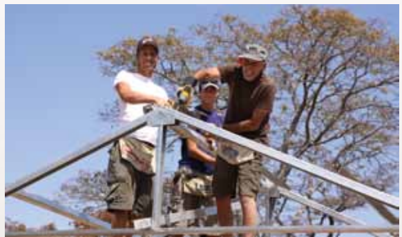
Caleb Knowles, Zack Barrow, and Steven Grabiner work on the roof of a church.
