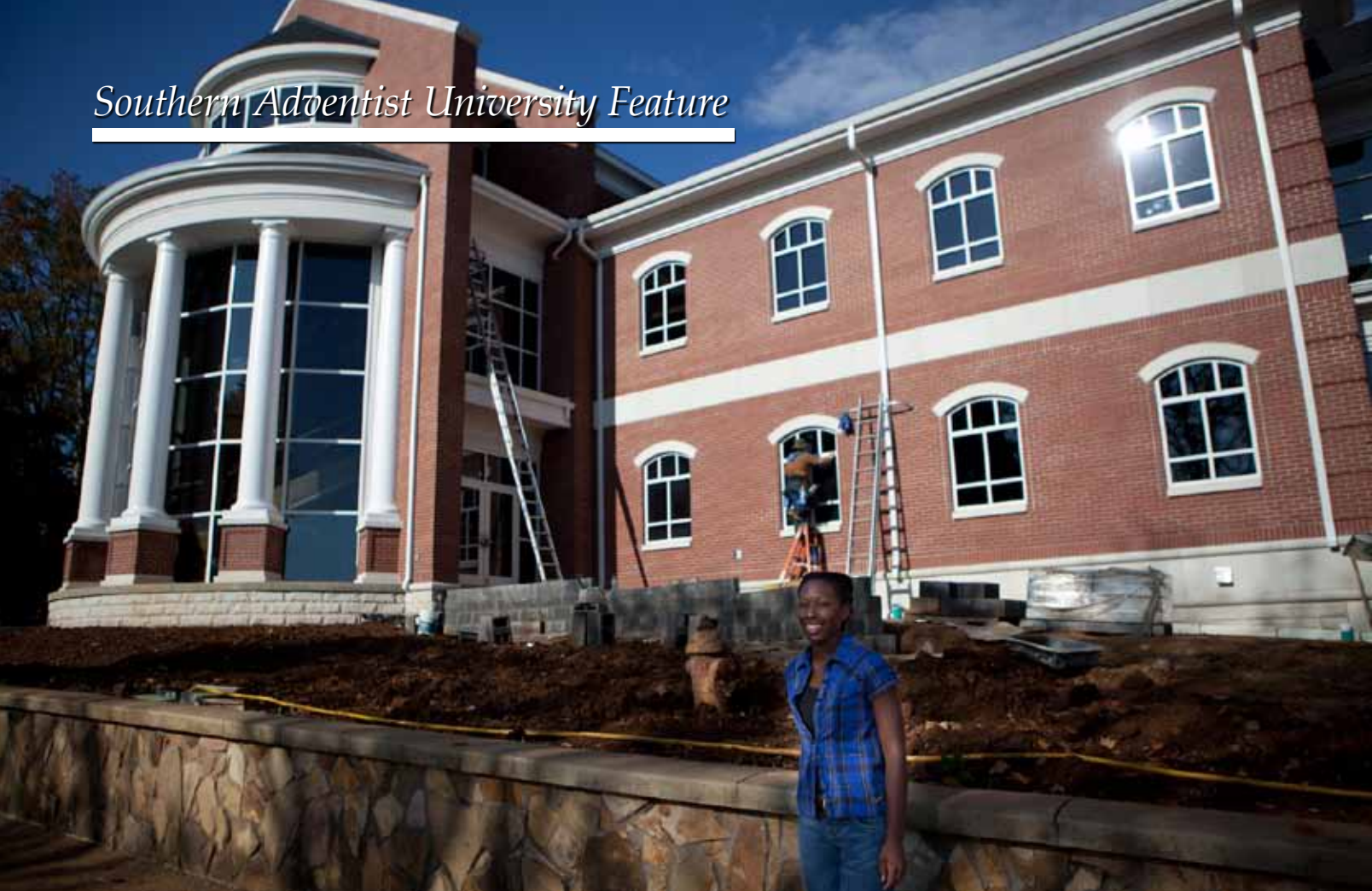
As construction wraps up on Florida Hospital Hall, Jonika Freeman dreams of the day she will be able to take classes in that building.
