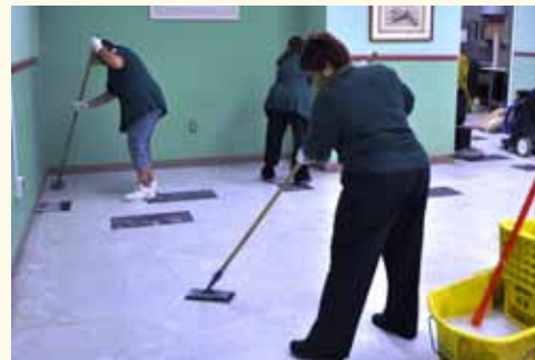
Martha Tremblay (left), Estelle Schiavo, and Joyce Lunsford work hard to scrub the floors, removing the old finish so that a new finish can be applied.
