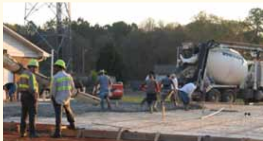
Loganville Church sanctuary foundation being poured. The church celebrated the opening of this new sanctuary on August 20, 2011.
