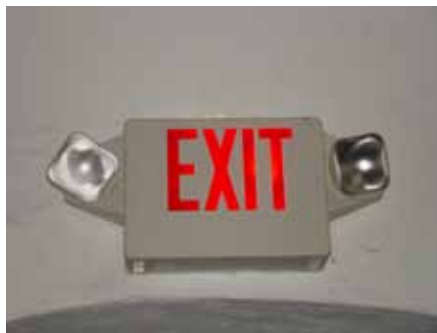
All exit signs should work properly — no blown bulbs.
