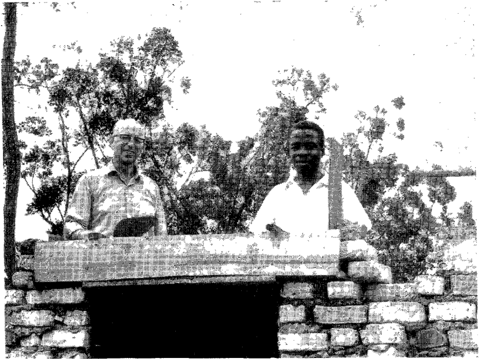
Volunteer layman, Louis Thayer (left) of Minneapolis, Minnesota, U.S.A., laying sun-dried bricks for the new classrooms and administrative buildings for Gitwe College in the Republic of Rwanda.
